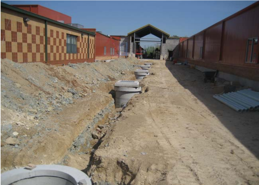
Courtyard area storm drain piping
