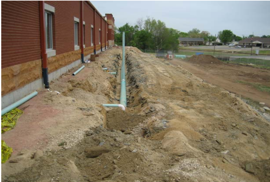
Storm sewer piping connecting downspouts
