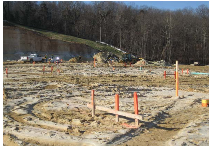
The building layout marked with batter boards. Crews excavate footings in the background
