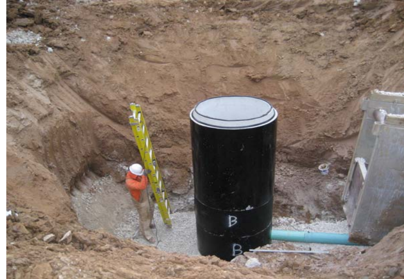
MH-B on gravity sanitary sewer; roughly 4-5' of rock broken out with breaker to set structure.
