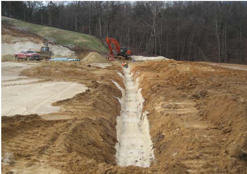
8" water main excavation on the north side of the building from fire hydrant at NW corner of building pad.
