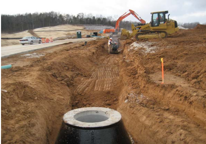
December 1st - Work begins on Site Pkg. #2 installing 8" gravity sanitary sewer from MH-A in foreground back toward MH-B.
