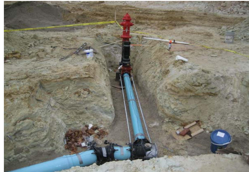
8" fire water main around the building; fire hydrant installation at SW building corner.
