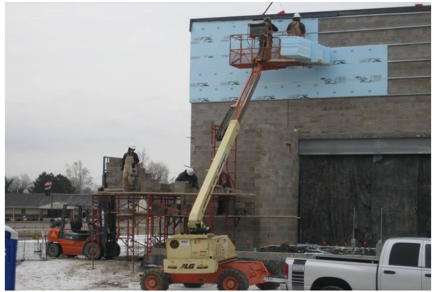
December 30th - Snow falling as masons work on CMU walls at the west elevation of building. Carpenters install insulation board and "Z"-furring for metal siding.
