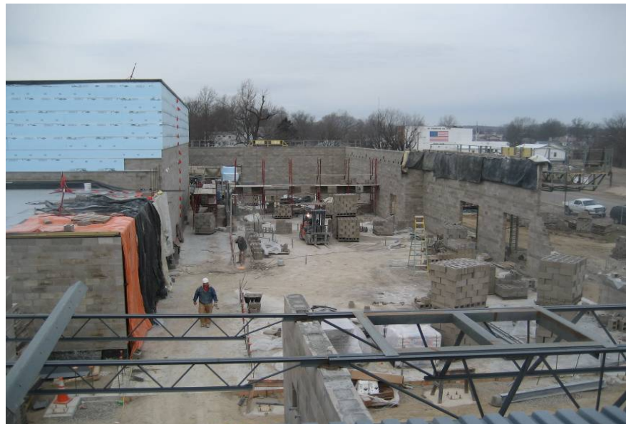
January 27 - Progress on CMU walls in the fine arts area. Work started on interior load bearing CMU walls and shear walls
