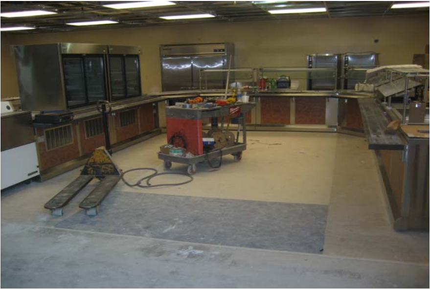
New kitchen serving line
