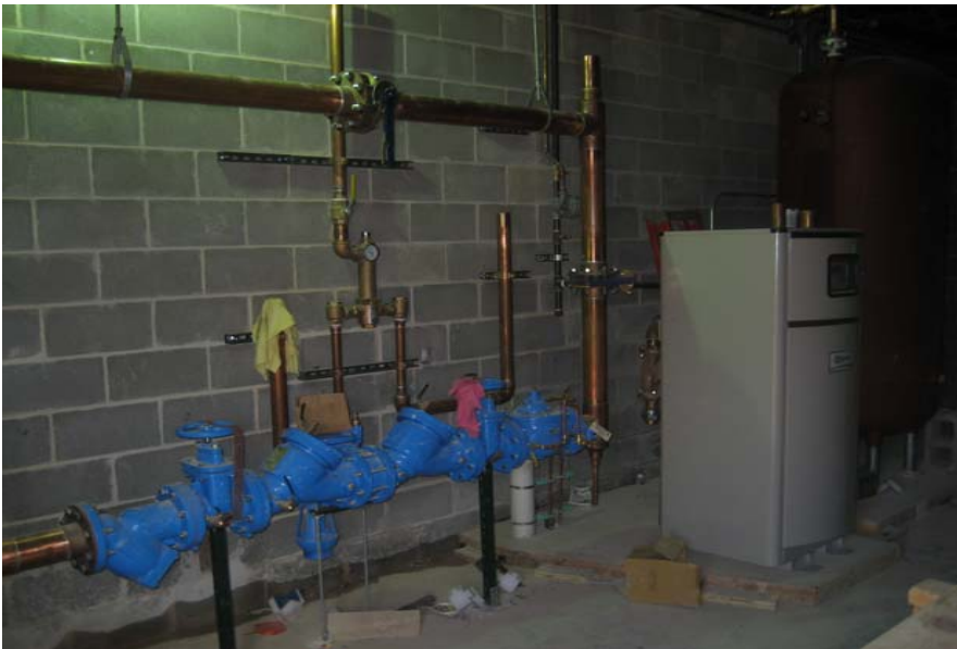
Main water service into building
