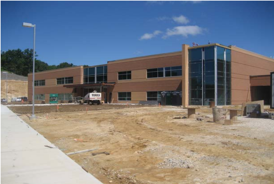
Building exterior in mid-July with walks poured & job trailers moved off site
