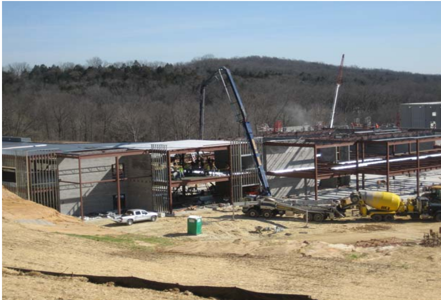
March 20, 2009 - Pouring the 2nd floor slab on deck west third of A building
