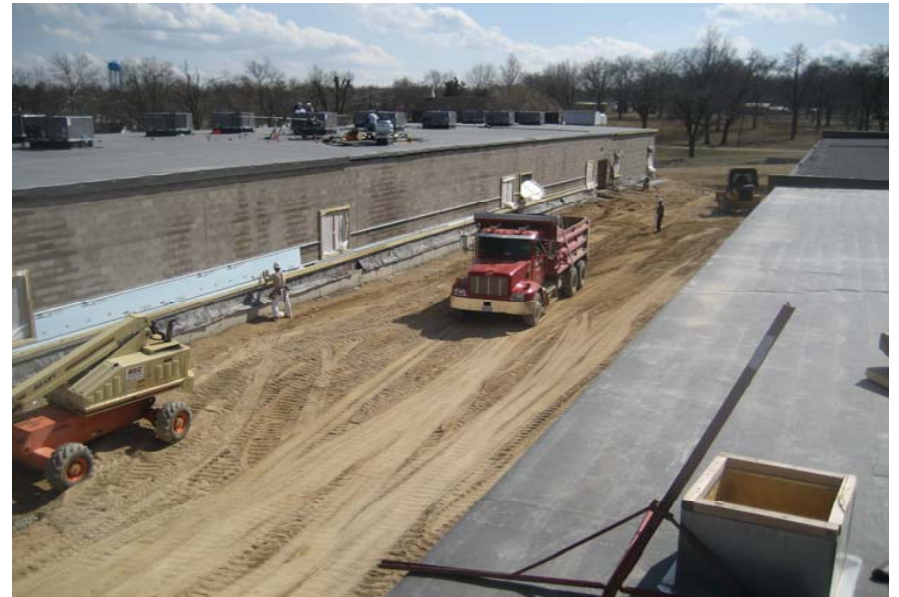
Fill installed in courtyard area; work on stone courses and wall insulation
