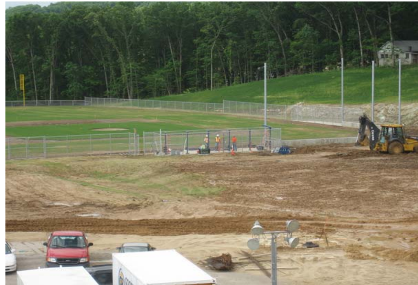
Dugout structures installed at baseball field; sod infield installed, seeding of outfield complete, irrigation system operational
