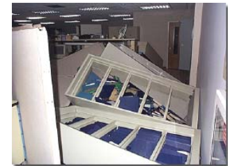
This example of non-structural damage is common after earthquakes of even moderate size - © FEMA File Photo
