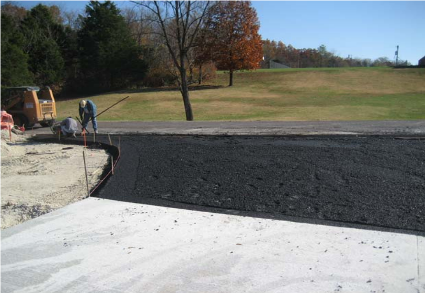
Asphalt paving of entrance off Dooling Hollow Road to new concrete pavement.
