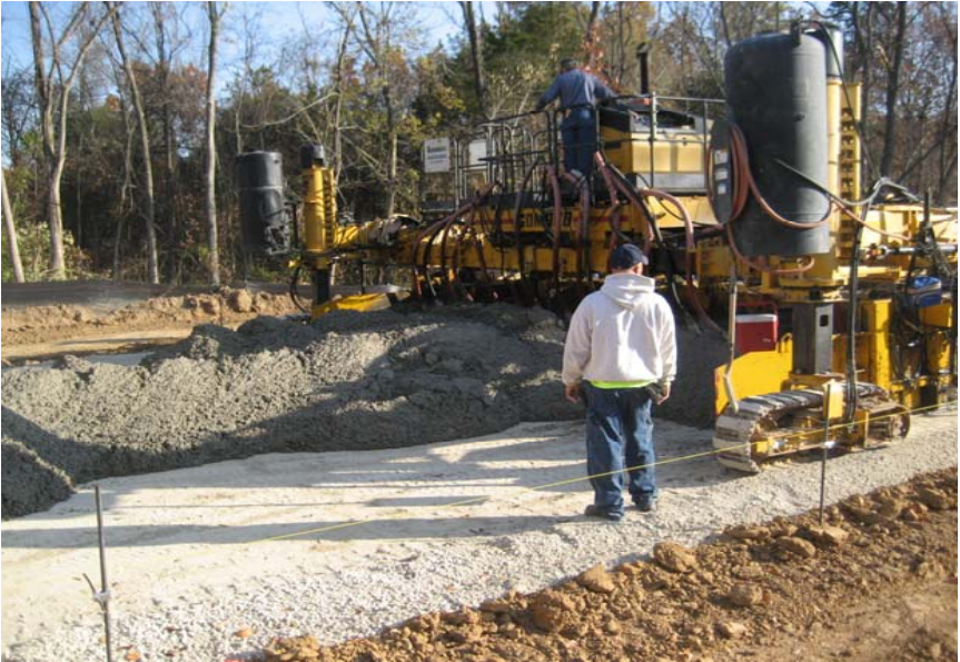
Paving operations, concrete dumped in front of paver, machine spreads concrete to laser control operation from grade string.
