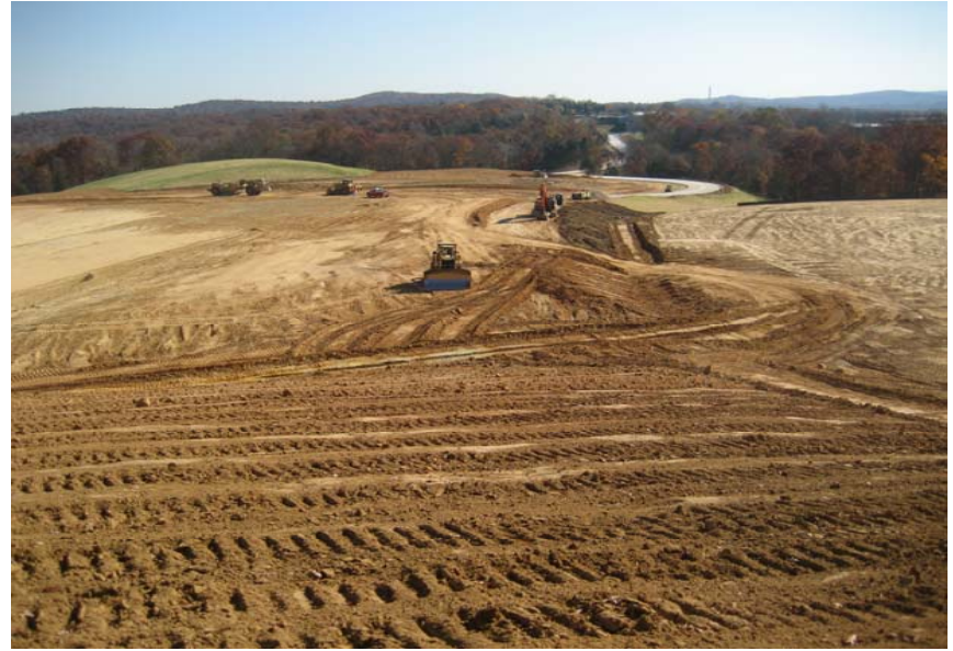
Finish cuts at west slope to complete fill in east parking lot.
