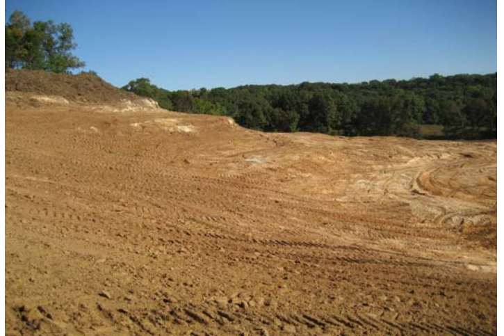
West slope of site starting to expose sandstone ledges; top of slope is roughly 66 feet above finish floor elevation.
