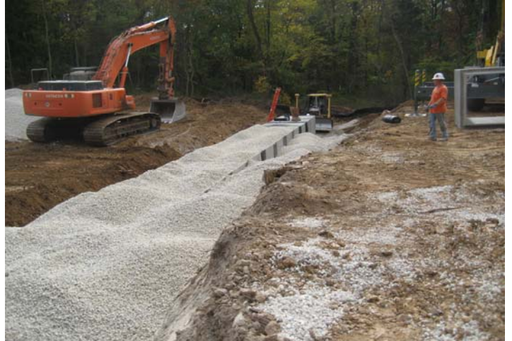
Box culvert installed and rock backfilled ready to install dirt fill for new main road entrance to High School site.
