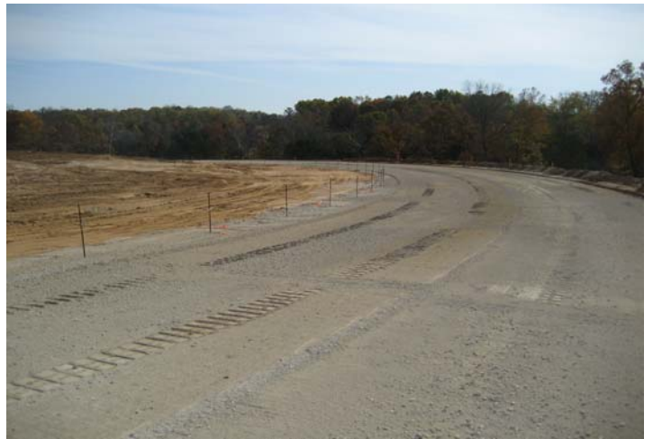
Main entrance roadway rock trimmed for paving, paving grade sting installed. Concrete paving to be done Nov. 3rd.
