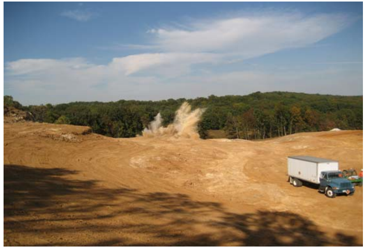
First blast shot of sandstone from west slope, 51,000 cubic yards of sandstone were shot and placed as compacted fill.
