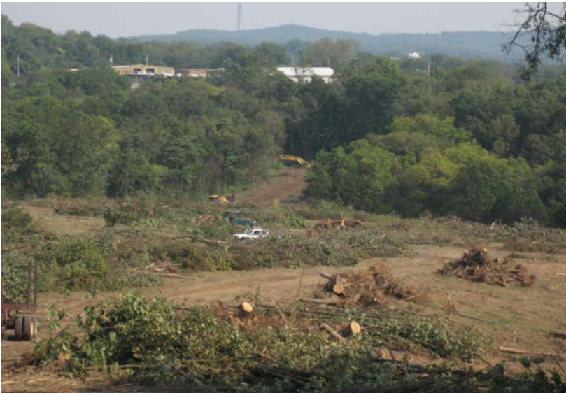
Day 4: Sept. 22nd, clearing timber east portion of site and new roadway to site.
