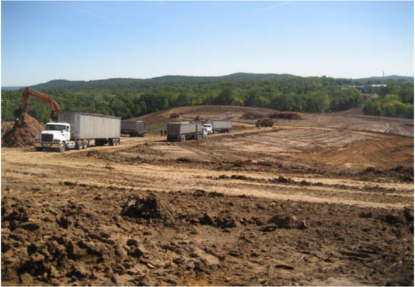
Day 11: Sept. 30th, Hauling chipped timber from site, cut & fill work progressing at baseball field, topsoil stockpiled.
