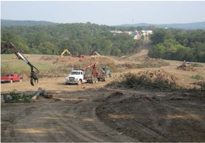
Day 7: Sept. 25th, New Roadway cleared, chipping timber east portion of site, loggers removing usable timber.
